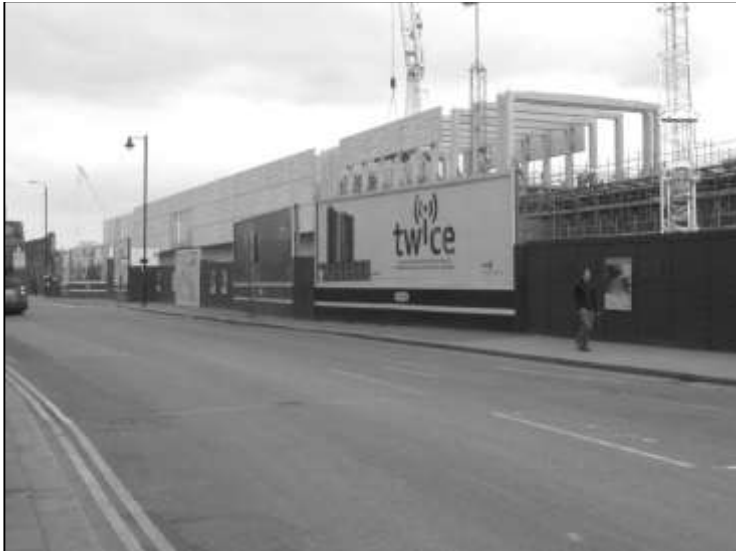
Left: Construction of the East London Line extension proceeds. On 16 September 2008 the superstructure of Shoreditch High Street station was well in evidence alongside Bethnal Green Road. The concrete boxing in of the line is being taken as far as the bow-string bridge over Shoreditch High Street to acoustically isolate the line from future building developments.
