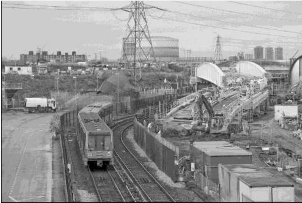
The new DLR flyover under construction east of Canning Town which will carry trains from Bank/Tower Gateway to the Beckton branch over those towards the Woolwich Arsenal line. This view was from Silvertown Way on 22 January 2009.
