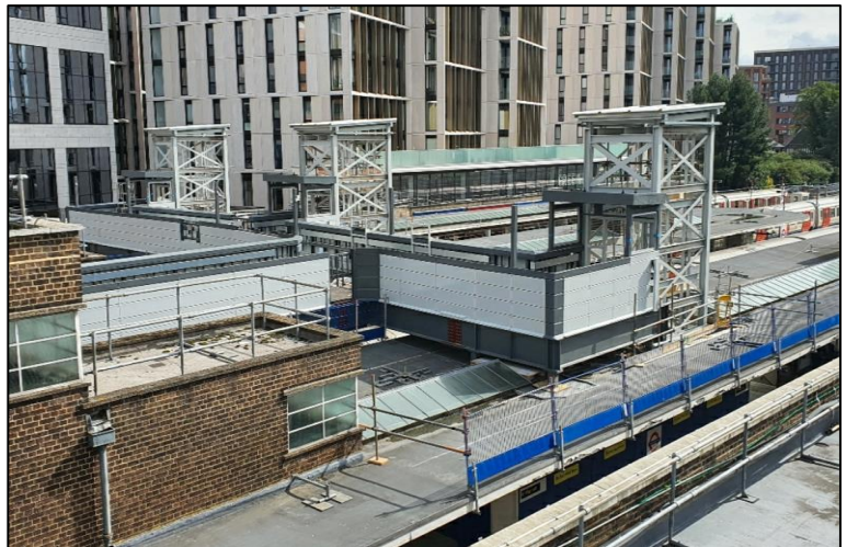
Above: Looking across the station canopies with the installation work in progress.
