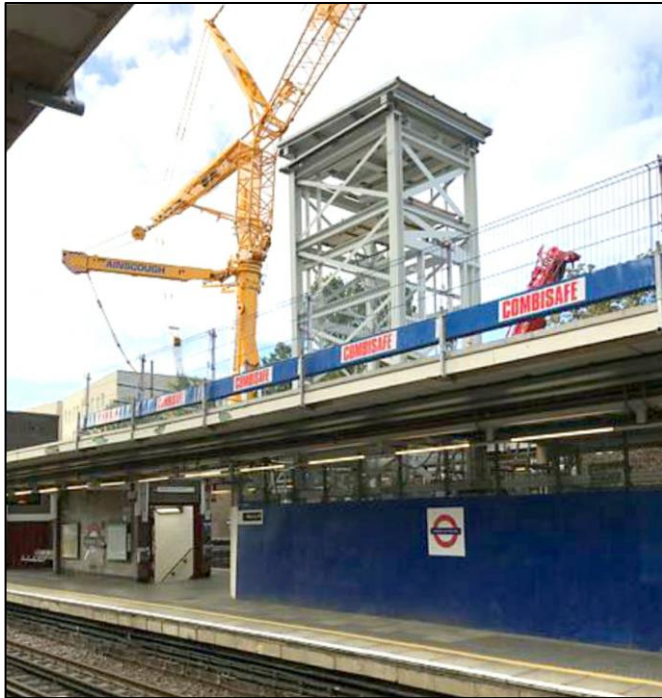
Above: Seen on 18 August 2020, the first lift tower 'shell' on platforms 3 and 4 is seen in position at Harrow-on-the-Hill.
